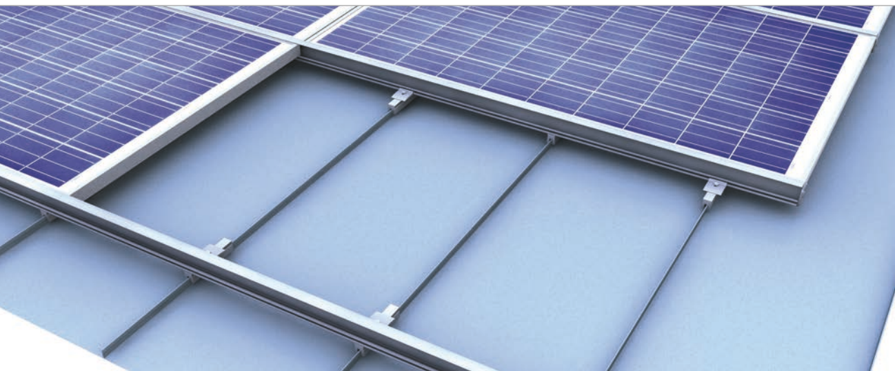
Single-rail insertion system with modules installed in landscape
