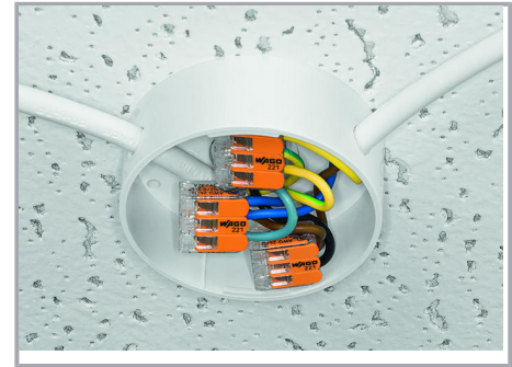
Lighting distribution in a ceiling canopy
