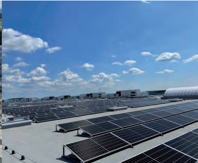
ŚWIEBODZIN, capacity 1,8 MW , structure type: DP-DNHBE- 15°, DP-DNHWE - 15°
